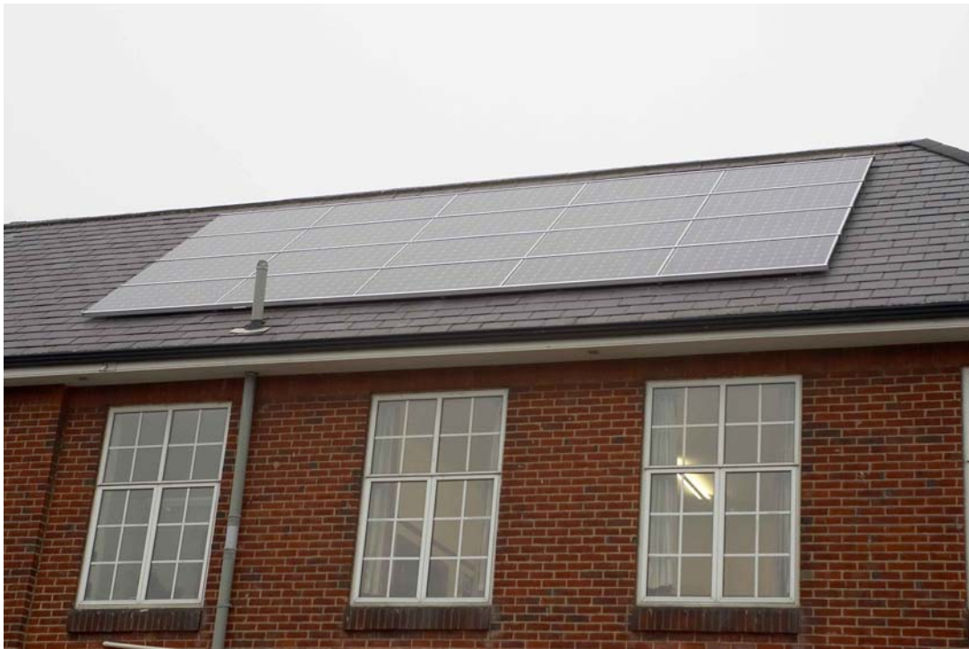
The solar panels on the roof of Farnborough Community Centre
